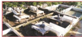
Surface Aeration Type
