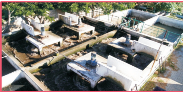
Surface Aeration Type
