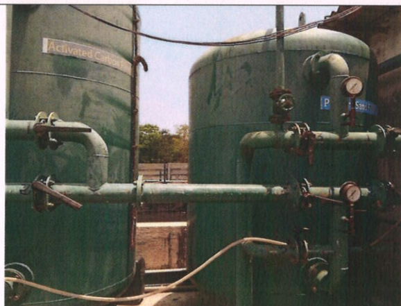
Fig8: pressure sand filter and activated carbon filter
