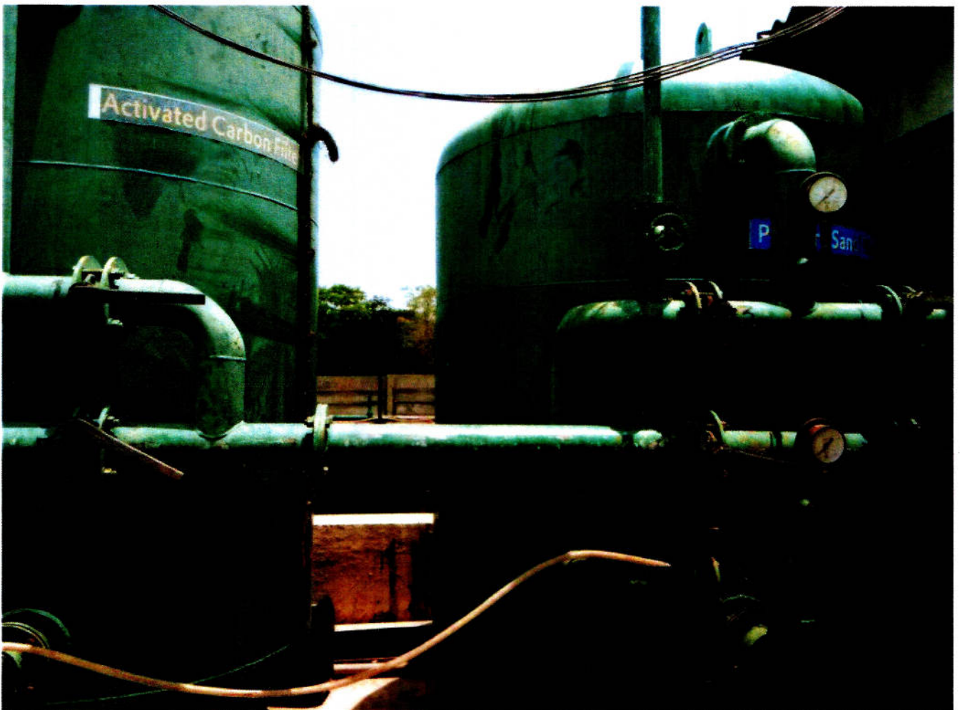
Fig7: pressure sand filter and activated carbon filter
