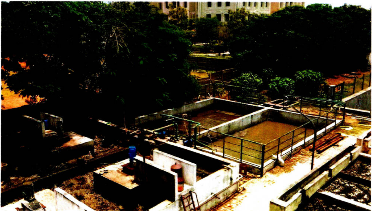
Fig2: overview of the collecting tank
